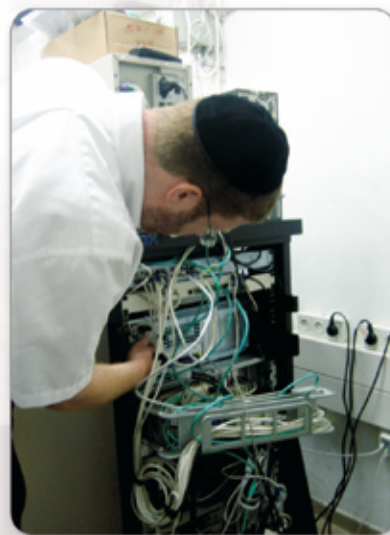
The Open-E NAS is connected to the campus-wide network of the Bar Ilan University by Fast Ethernet.
